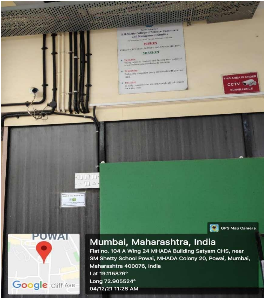
CCTV Camera installed at each floor (above pic &th floor)
